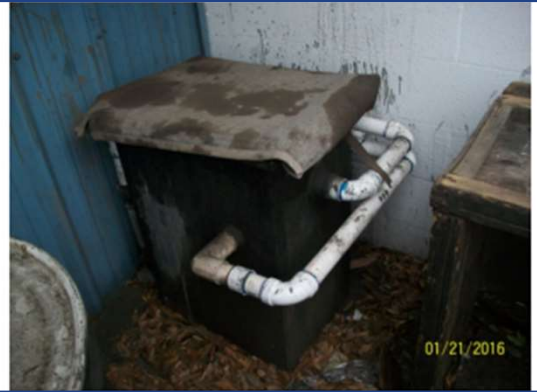
Photograph 7: Plumbing from sink leads to this settling tank.
